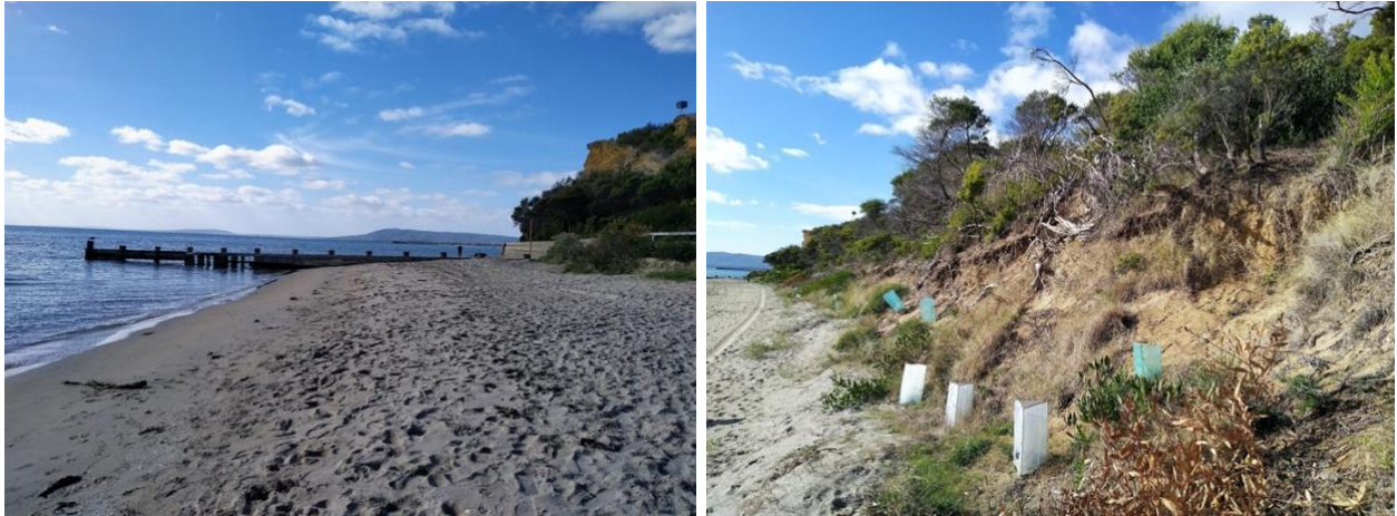
Tyrone Foreshore. Left: Hole evident in the groyne, increasing sand erosion. Whitecliffs Lookout can be seen in the top RHS. Right: Due to potentially rising sea levels and increasing tide surges, the reserve edge is gradually eroding. Planting of salt bush has been partially successful; some died but surviving plants take off quickly and bind the “soil”. Photos S Richards.
