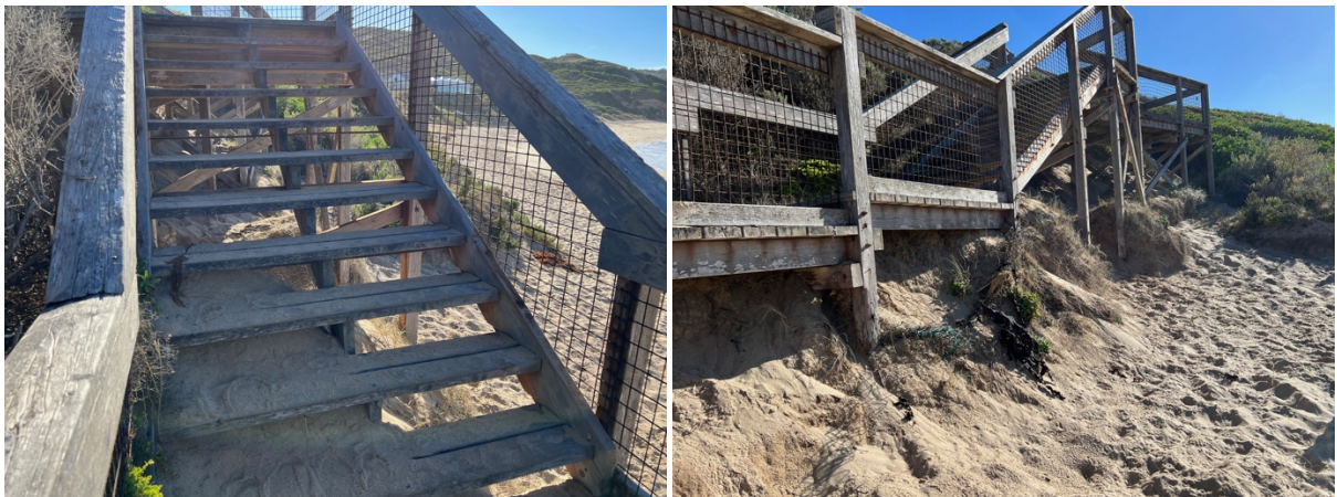
Sorrento Back Beach - dune erosion under the stairs where all vegetation has been removed. The indigenous coastal vegetation seen here to the right of the stairs is critical to holding the cliff and dune in place. Photos U de Jong
